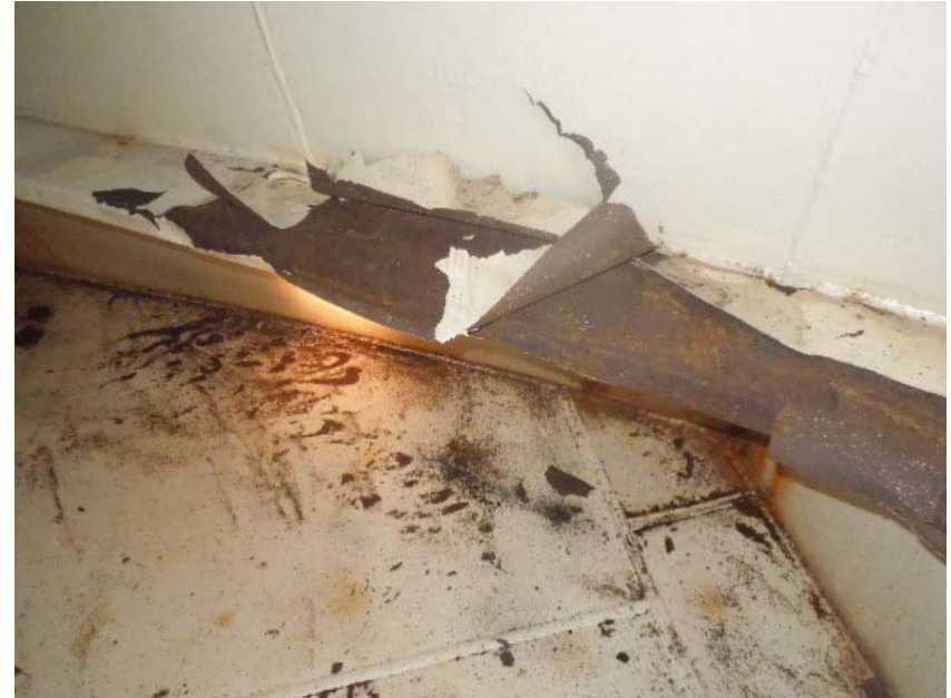
Severe coating breakdown within 2 years of coating in accordance with PSPC.
