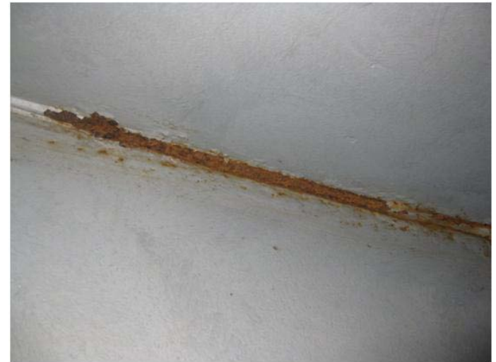
Example of inadequate stripe coating leading to breakdown
