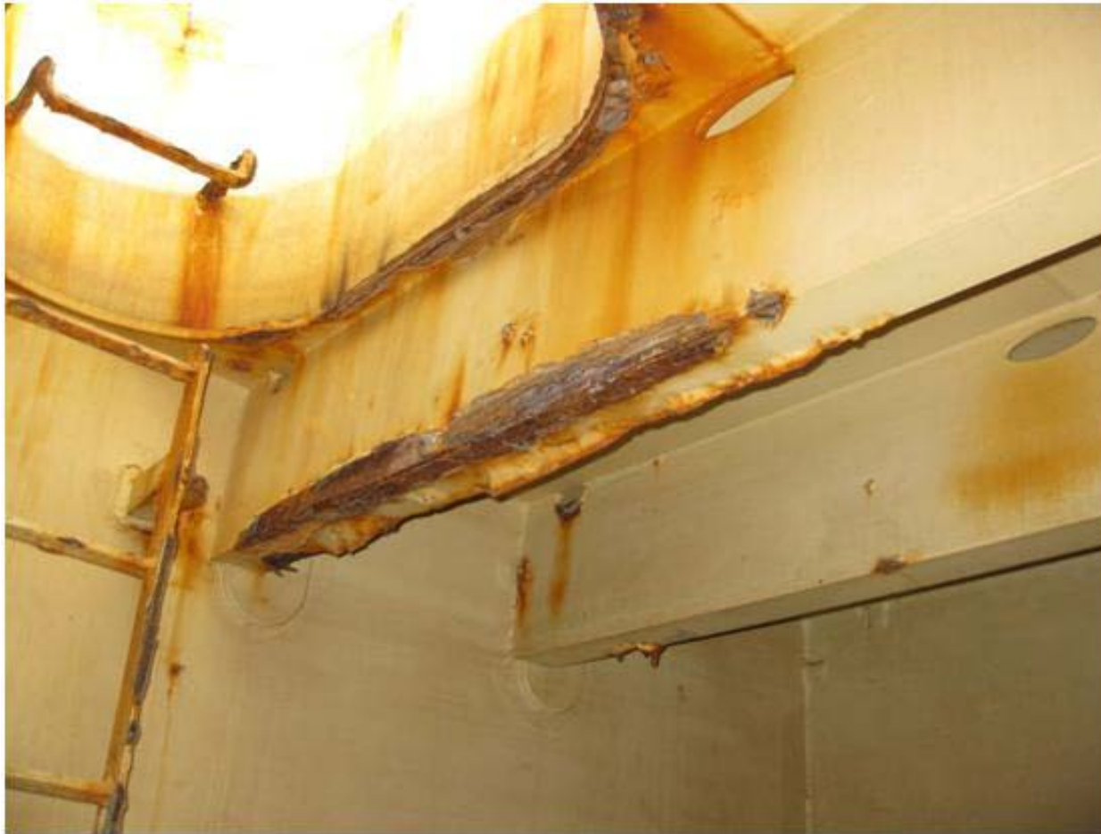
10 year old ship with coating breakdown on access ladders, coaming and longitudinal edges due to insufficient stripe coating and poor treatment of non-integral fittings
