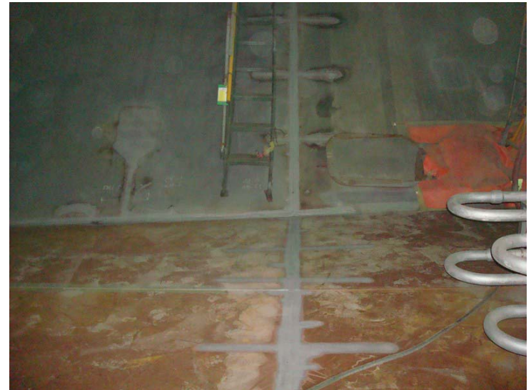
Example of poor BHP performance
